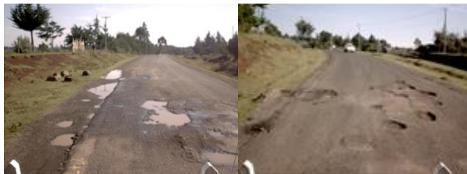
Figure 2: Major distress and lack of defined system
