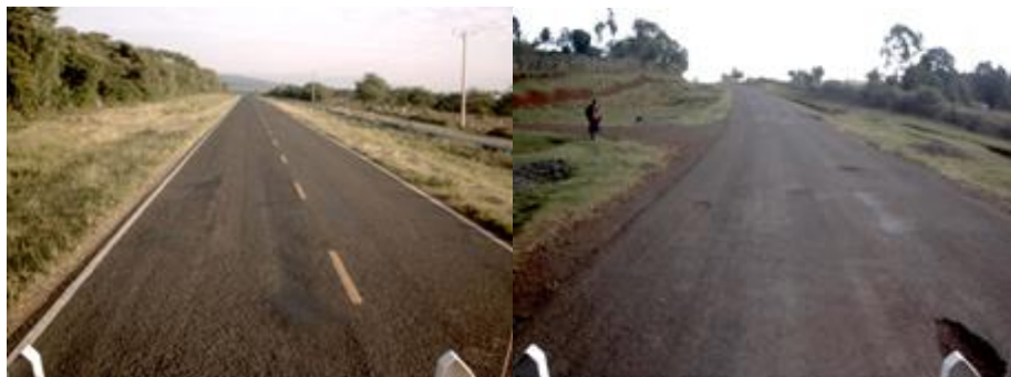
Figure 1: Minor distress and lack of drainage system on Kampi ya Moto-Kamwosor Road
